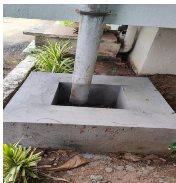
Figure 5: Vertical discharge pipe and discharge
